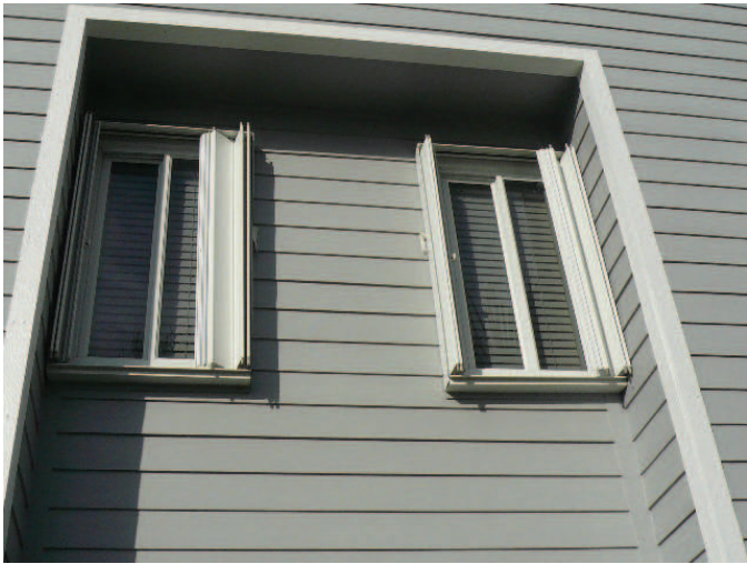
Non verified shutters
