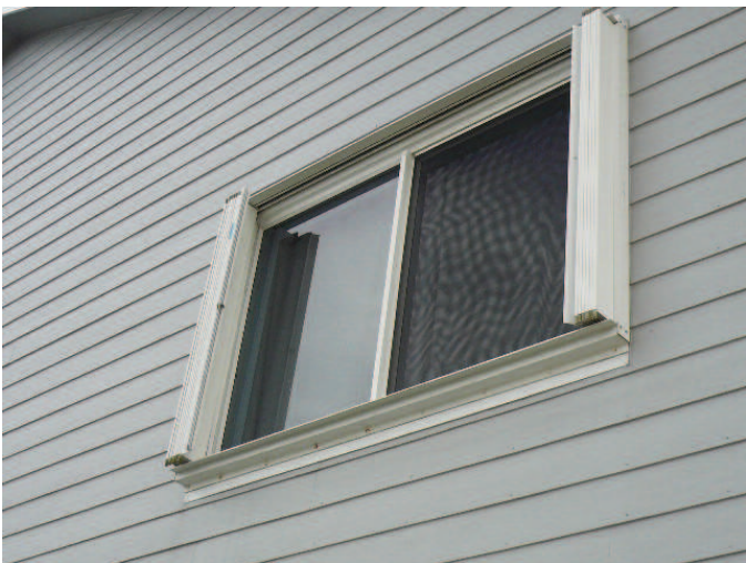
Non verified shutters
