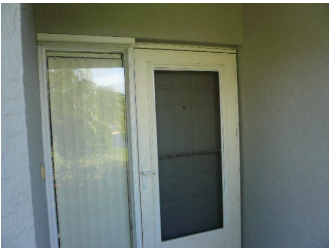
Door not shuttered or labeled as impact rated
