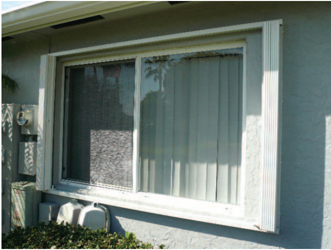
Non verified shutters
