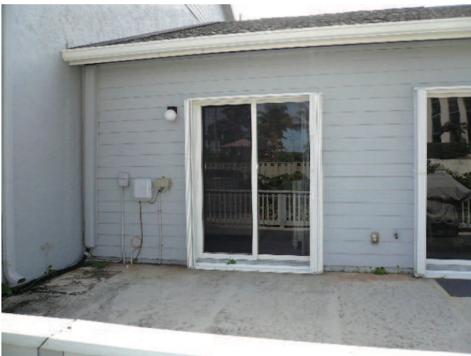
Non verified shutters
